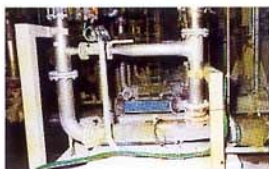
Application: coating kitchen. Seven seepex pumps BN 52-6L with dry running protection TSE 120 and flushing connection. Product: calcium carbonate, flow rate: 24.5/34.5 m 3 /h (108/152 gpm), speed: 171/238 rpm, pressure: 6 bar (90 psi), temperature: 5 - 55° C, spec. gravity: 1.9, solids content: 65 - 75% wt, viscosity: 1000 - 2000 cps
