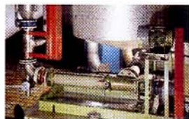
Crystallization Four seepex pumps BN 35-6L, product: high and low green molasses, flow: 4-25 m 3 /h / 18-110 usgpm, speed: 50-280 rpm, pressure: 2.7-3.2 bar / 40-45 psig, temperature: 70-85° C / 158-185°F, solids: 60-70% ds
