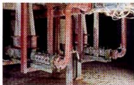
Juice Purification under a rotary vacuum filter. Three seepex pumps BN 10-12 and BT 17-6L with adjustable stator retensioning device, product: carbolime, flow: 1.7 and 6 m 3 /h / 7.5 and 26.5 usgpm, speed: 70 and 120 rpm, pressure: 3 and 6 bar / 43 and 85 psig, solids: 40 and 50% ds
